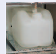
Condensate reservoir on pressure plate for automatic notification
